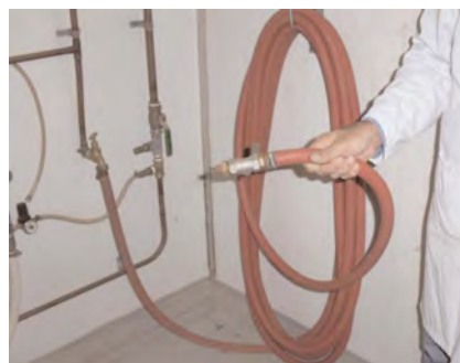
A hose left unattended for a total of an hour a day can waste as much as $3200–$6400/yr.
