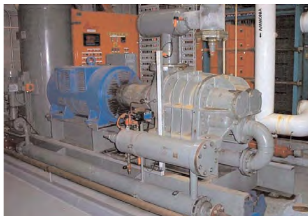
The compressor is the workhorse of a refrigeration system and usually accounts for between 80% and 100% of the system's total energy consumption
