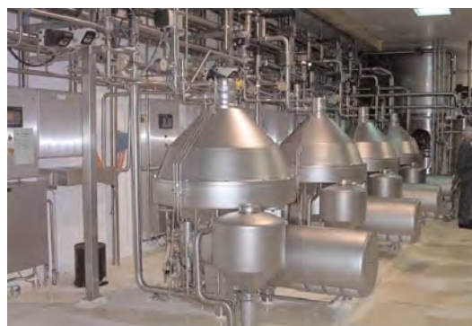
Optimising de-sludge frequency for all processes that utilise centrifugal separation of liquid milk streams will ensure that losses of milk components are minimised.
