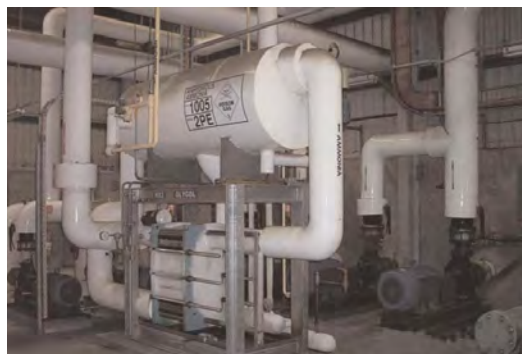
The cost of operating a refrigeration system can be up to around 20% of total energy costs in a dairy processing plant.
