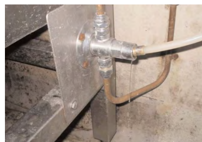
Taking supply water meter readings during non-production hours can highlight any unusual water consumption or leaking pipes.
