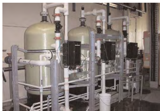
The treatment of boiler feedwater will help to minimise build-up of scale, which acts as an insulator and inhibits heat transfer.
